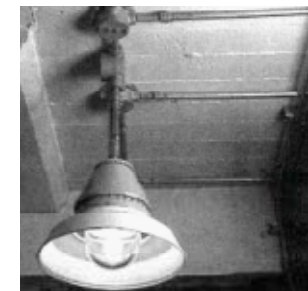
Typical Class 1 Div 1 conduit installation
